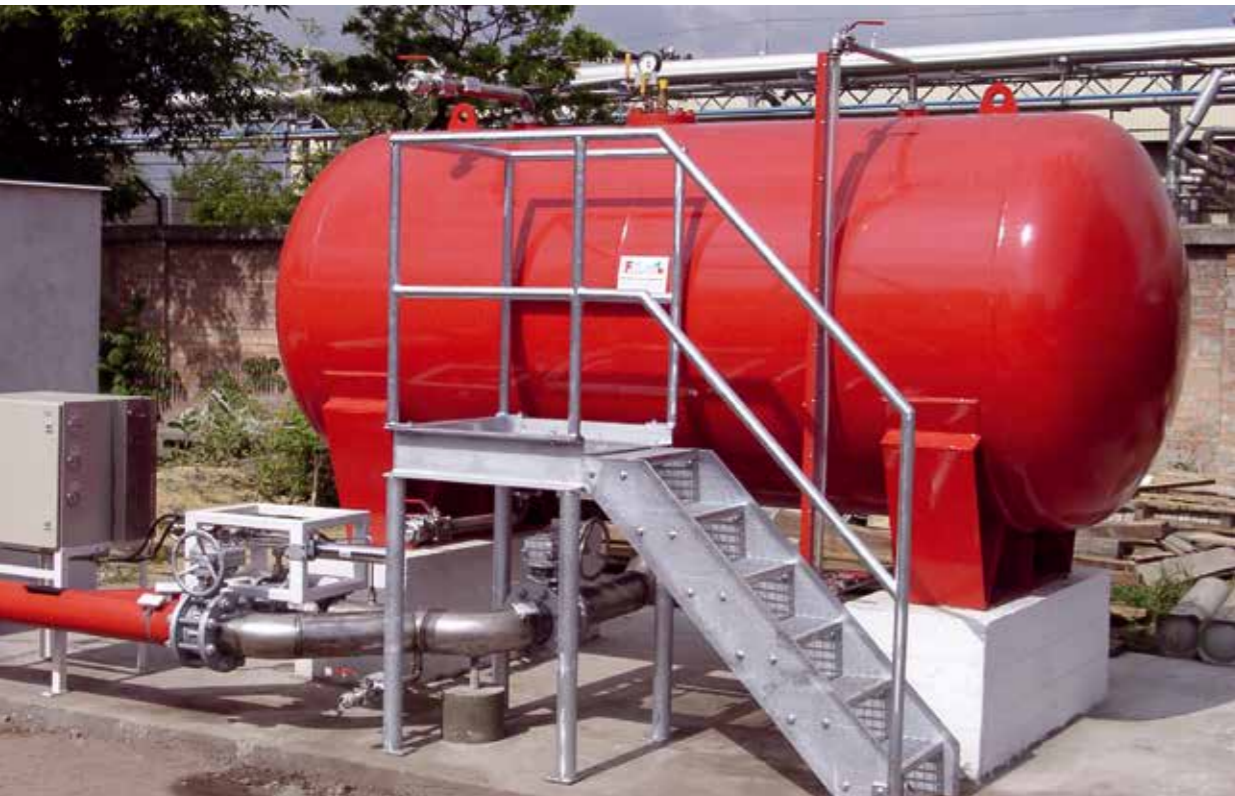
◀ A typical above-ground Pi Foam pressure vessel. Today, the bigger ones are almost always stored underground.
